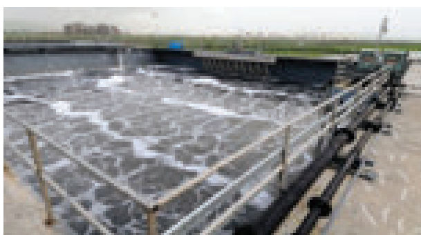
Figure 22.4 A view of sewage treatment plant
