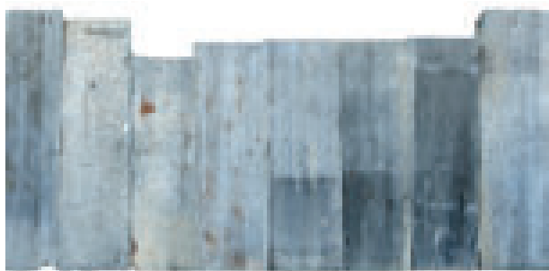
Fig 10.7 Damaged iron sheets
