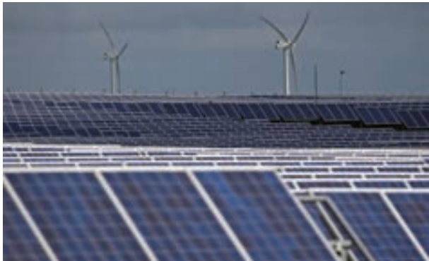
Kamuthi solar power plant
